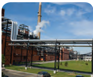
Onsite Utility Company
